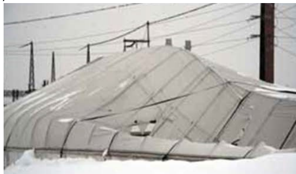
Figure 10: Peak-style high tunnel collapsed under heavy snow load, February 2010, Ithaca, NY.
