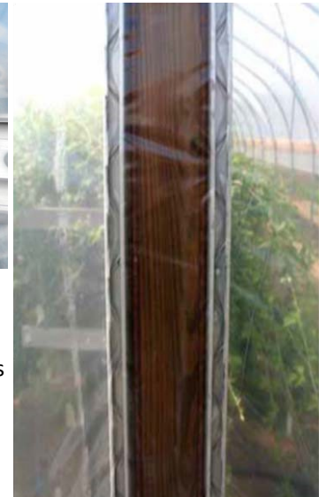
Figure 31: Plastic film attached to the end wall of a tunnel with aluminum extrusions (attached to the wooden frame) and zig-zag wire (wiggle wire). The zig-zag wire secures the film by holding it in place inside the aluminum (U-shaped) extrusion. The zig-zag wire can be easily removed when the plastic needs to be replaced. While the zig-zag wire can be used multiple times, it is often replaced when new plastic is installed.
